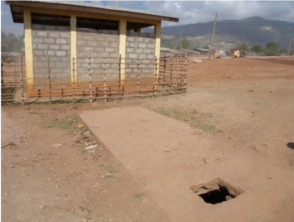
Ph. 27: Septic tank 2
