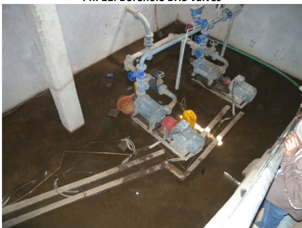
Ph. 13: Booster1: n. 2 pump sets
