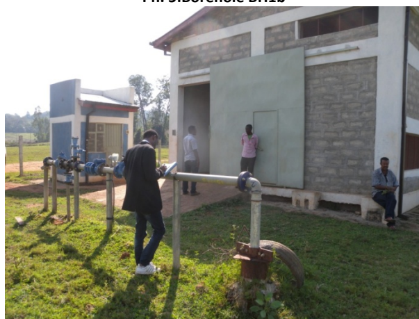
Ph. 7: Borehole BH2 and Pumping station
