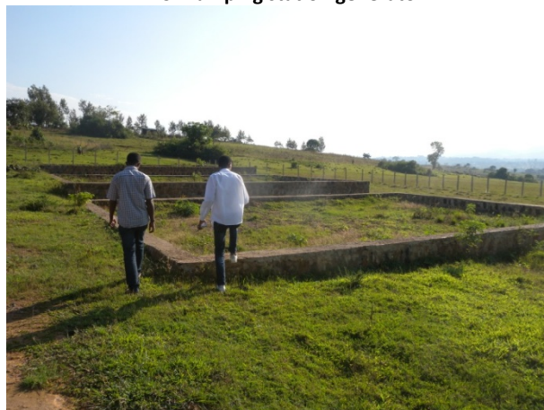
Ph. 11: Dry sludge bed
