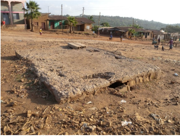
Ph. 25: Septic tank 1
