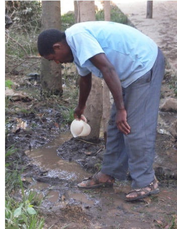
Ph. 28: Pipe break
