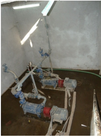
Ph. 21: Booster pumping sets
