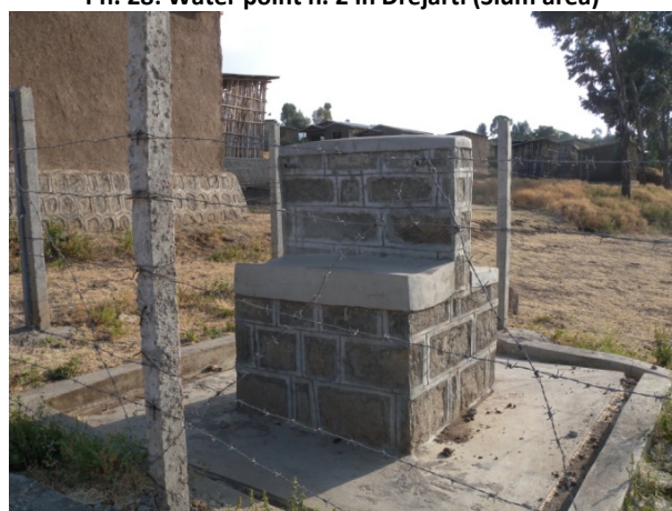
Ph. 30: Water point n. 5 (out of service)
