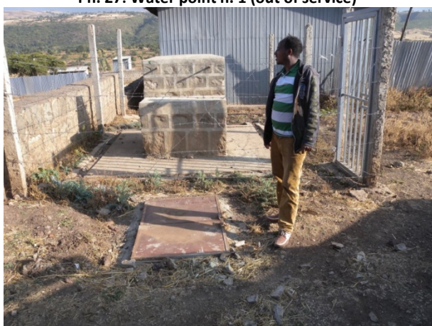
Ph. 29: Water point n. 3 (out of service)
