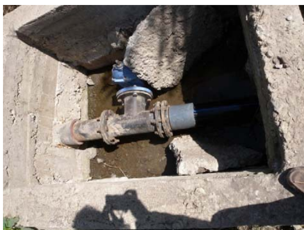
Ph. 25: Transmission pipe washout
