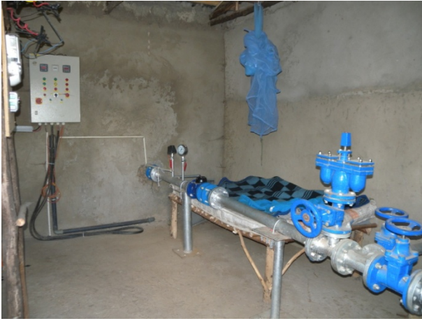
Ph. 17: Borehole BH4 valves
