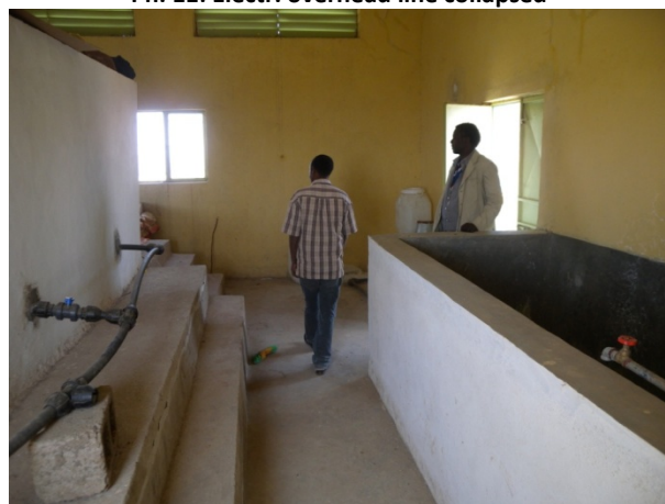
Ph. 13: Chlorization plant (out of order)
