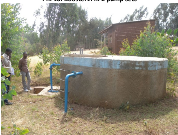
Ph. 15: Break pressure tank (BPT)
