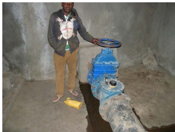
Ph. 24: Tank outlet DN 300 mm, to the town network
