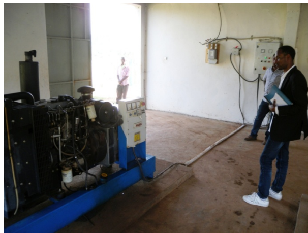
Ph. 9: Pumping station generator
