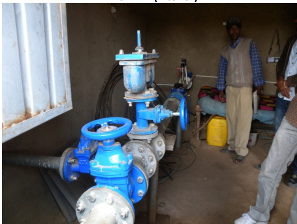
Ph. 11: Borehole BH3 valves
