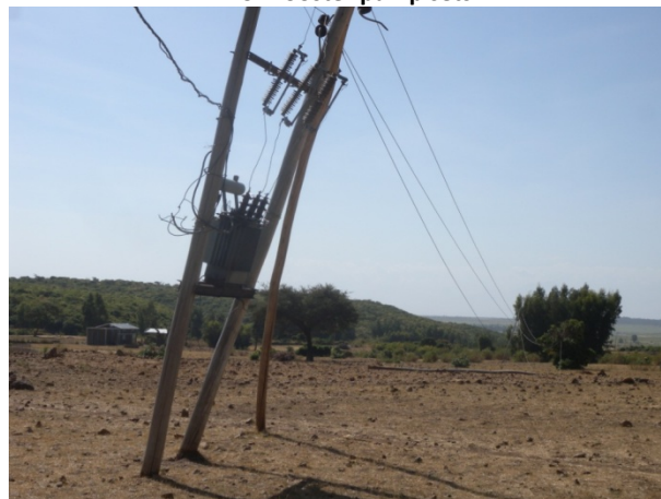
Ph. 11: Electr. overhead line collapsed
