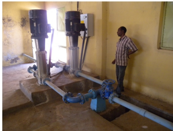
Ph. 9: Booster pump sets
