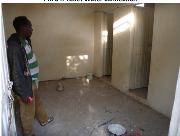
Ph. 36: Toilet showers
