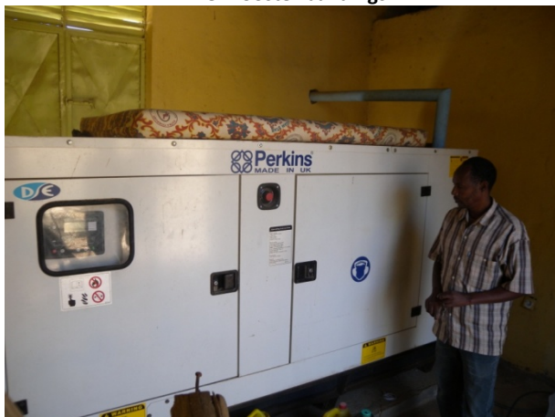
Ph. 10: P. generator
